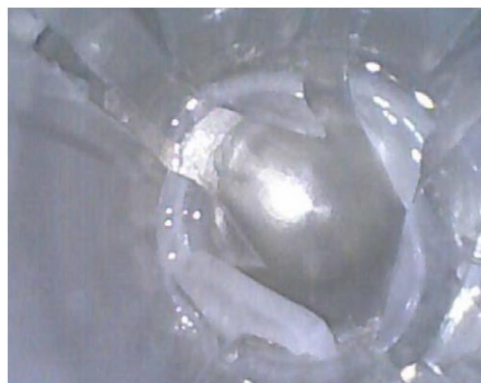
Example of a damaged internal plastic liner (bottom part)
